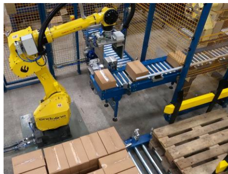
Image 2: The fully integrated, robotic palletising line, installed by Endoline Robotics, has dramatically increased efficiency while cutting time for the company
